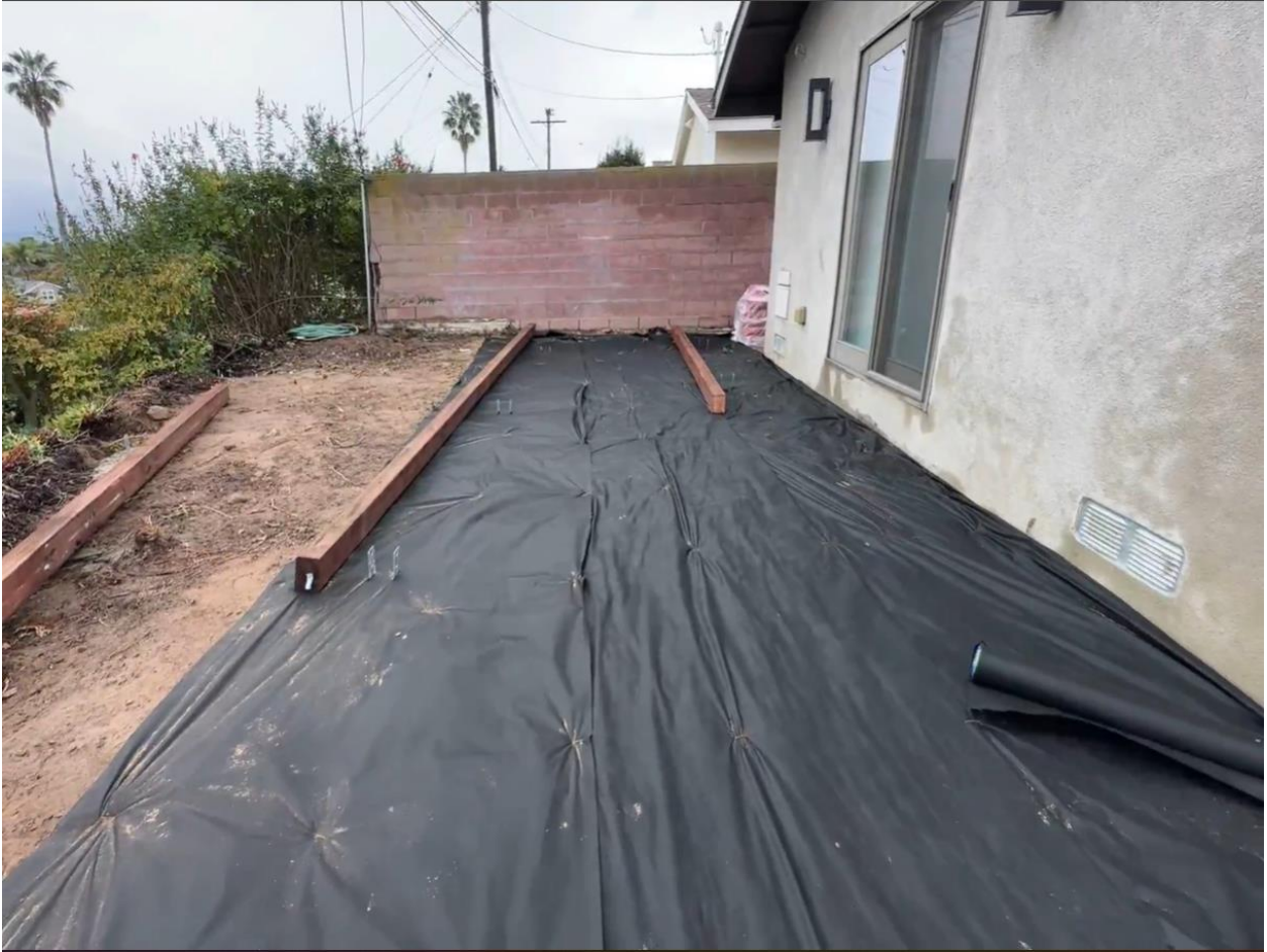
Photo 2B: 5608 White Ct during deck construction. Note: ground is level beyond cinder block wall to property line.
