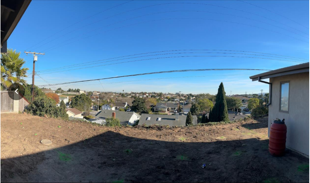
Photo 3B: 5608 White Ct during deck construction. Note: area greater than 10' and not part of 10' setback.
