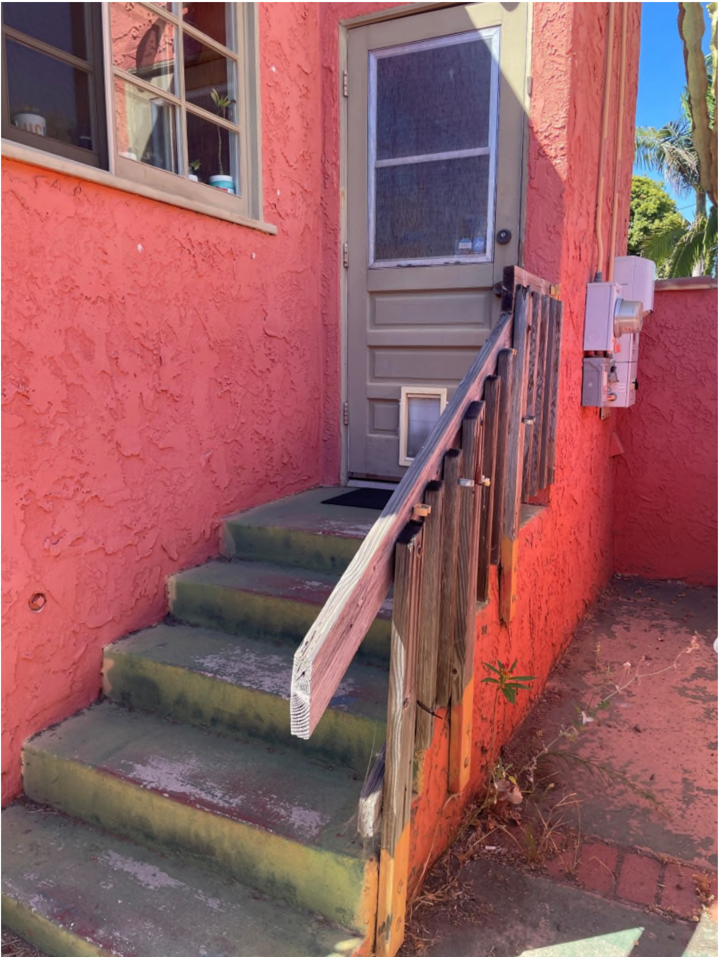
Rear kitchen door and stair railing
